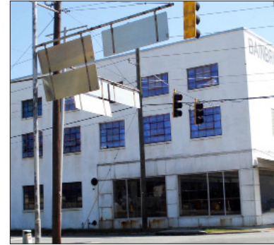
Upper windows on rears of buildings, mid-to-late-20th century buildings, or industrial buildings are constructed of steel mullions. Use rust-bonding primers, reglaze and paint to retain these character defining features.
