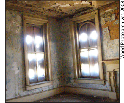
The oldest wood windows are especially salvageable. Fully rotted pieces should be rebuilt and older-growth hardwood can be oiled, primed, and painted. Covered windows may be found on upper floors.
